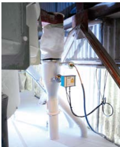
The Parsum installed in-line, on the take-off from the sieve stack.
